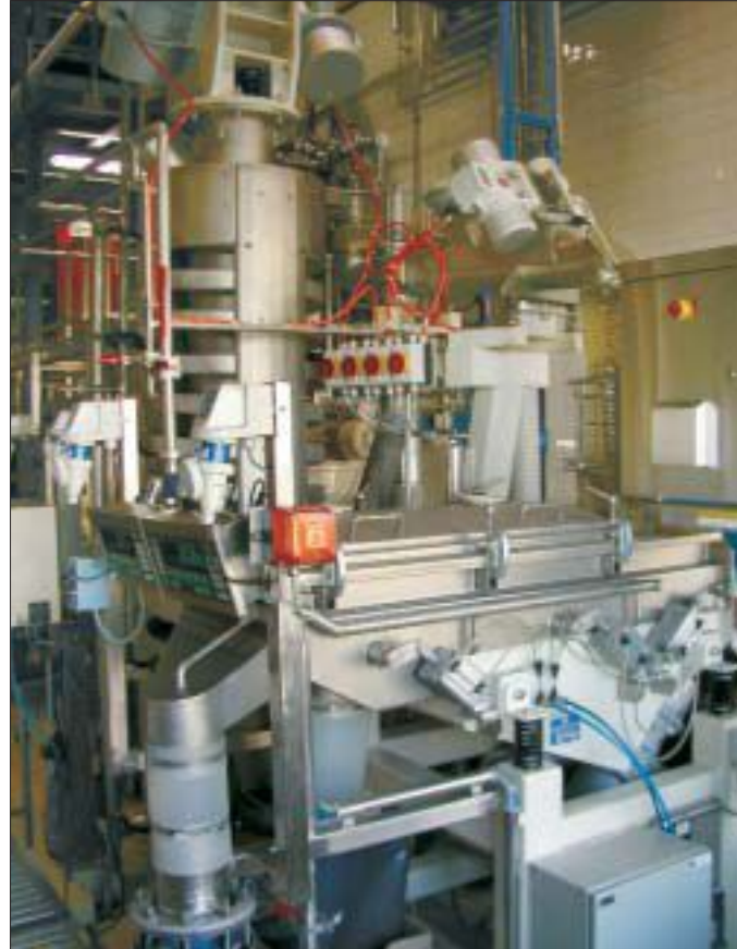
Figure 40 SR 15/6-I vibratory screening machine in a chemical plant
