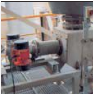
Figure 39 Vibratory screening machine handling 600°C hot bulk material
