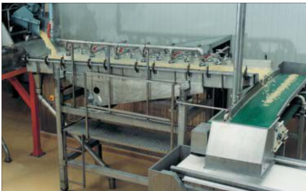
Figure 22 ESR 30/6 dewatering screening machine, 3000/600 mm, in a canning factory
