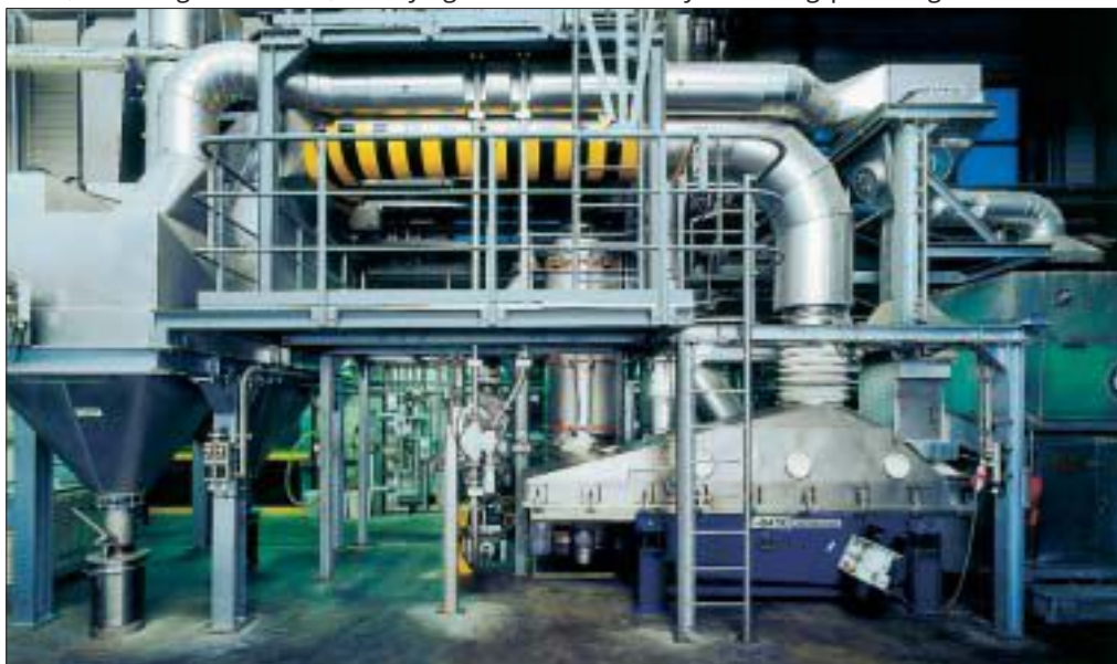
Figure 31 VSK 25-7/7 vibratory fluid-bed dryer with integrated screen and complete air-handling equipment, including a dust filter, for drying and simultaneously screening plastics granules
