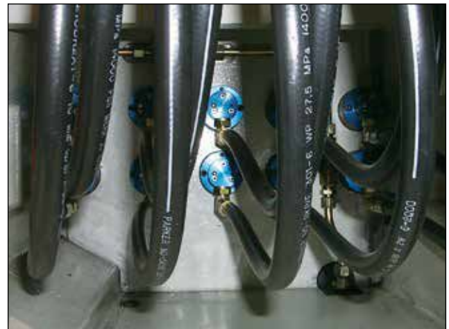
DEUBLIN 1117 Bearingless Unions on Automotive Transfer Line
